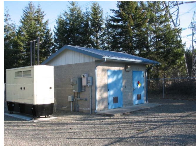
Sugarloaf Well #3 Treatment Facility
